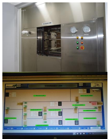
Autoclave and BMS
